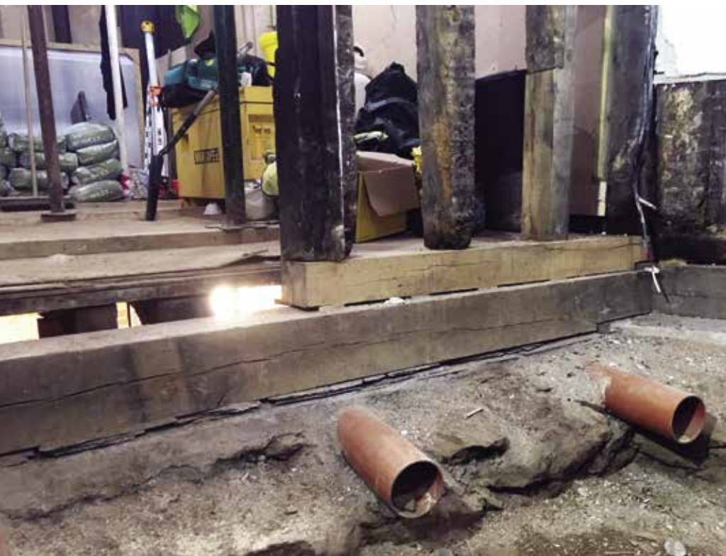
Above Oak sole plate repairs and ducts for radon protection on site
