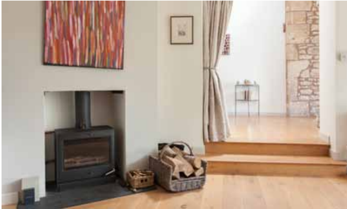
ABOVE: The couple put in the Stovax wood burner which heats a boiler, and this supplies the radiators on this side of the house
